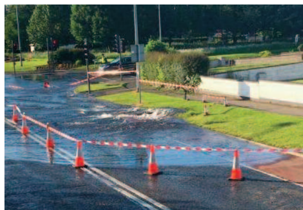
Burst mains water pipe, Leixlip, June 2019 image © Kildare Now
